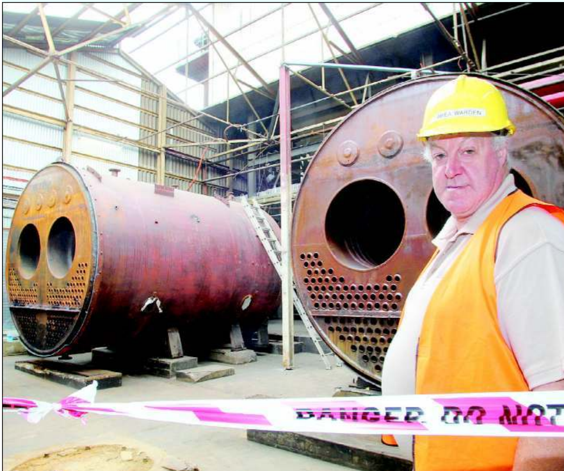
GREEN GOALS: Cascade general manager production Max Burslem oversees removal of old boilers from the factory. Picture: KIM EISZELE
